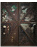
Rusted Metal Do...
